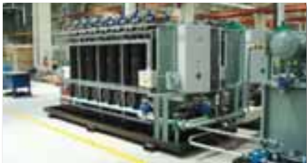
RS 2 treatment facility at OSS
